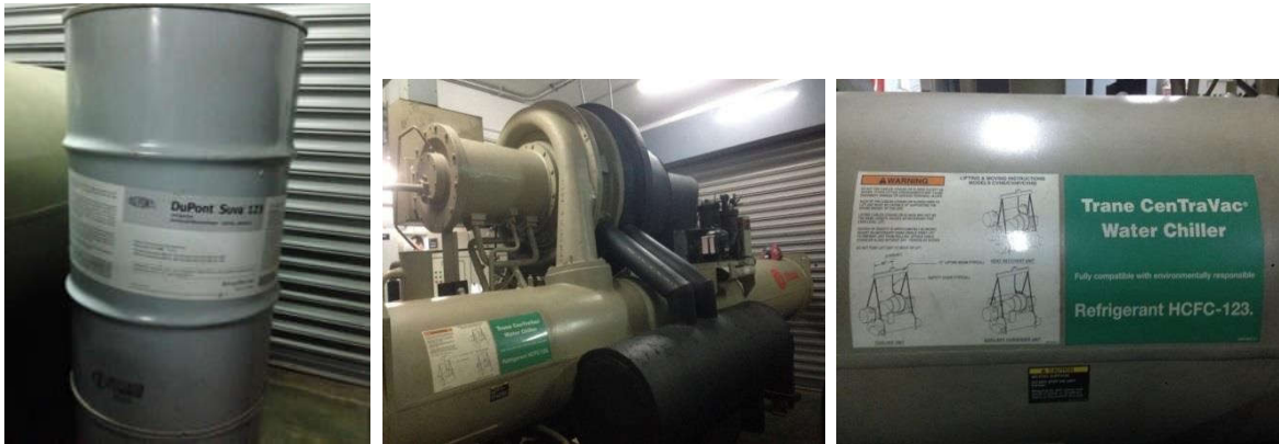
Figure 5 Non-CFC refrigerant, HCFC - 123 liquid refrigerant
